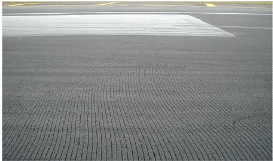
Figure 1.2 – Slippage at High-Speed Taxiway (“Curved” Grooves Indicate Slippage, Bognacki et al., 2007)
