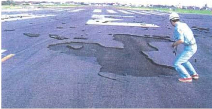
Figure 1.1 – Slippage Failure due to Loss of Bond at Nagoya Airport (from Tsubokawa et al., 2007)
